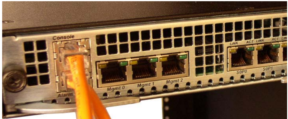
Figure 4 - 79. Console Cable Connected
