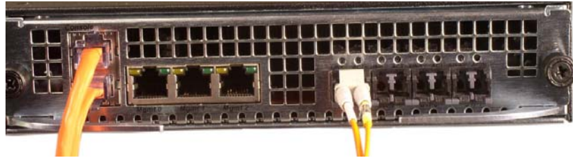
Figure 4 - 88. Connected S0P0 Optical Transceiver Connected
